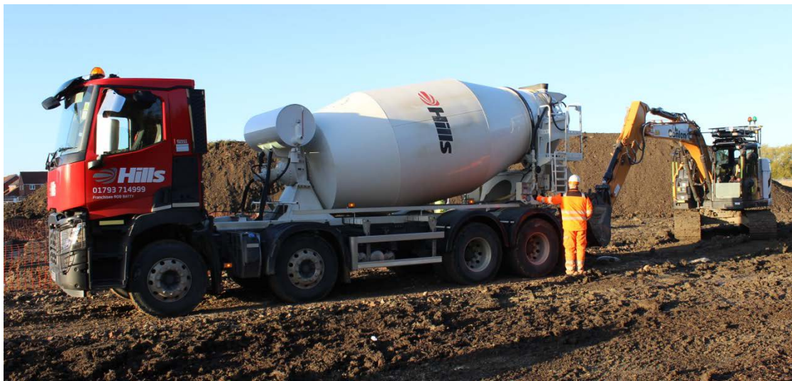
Hills Quarry Products' franchisee driver Rob Batty delivering Hills' 1.5millionth cubic metre of ready mixed concrete to customer Conlon's site near Wantage, Oxfordshire.
