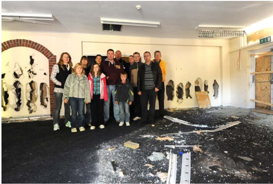
Residents survey the damage caused by vandalism inside the NAAFI building
