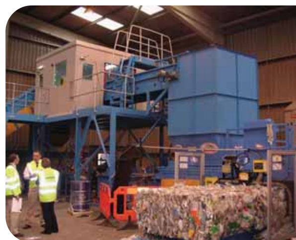
The new 'Badger' baler installed at the MRF
